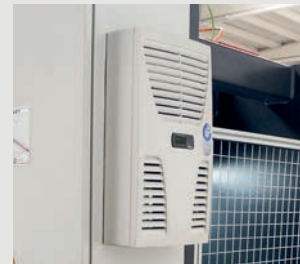
Electrical Cabinet Cooling System
